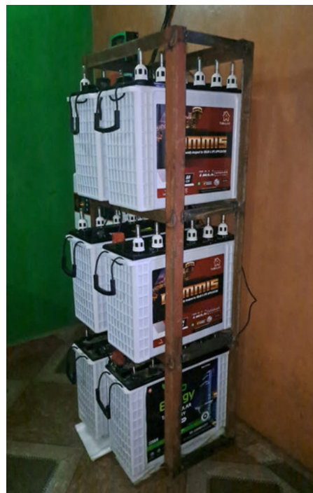
Batteries that store electrical energy generated by solar panels deployed on rooftops.
