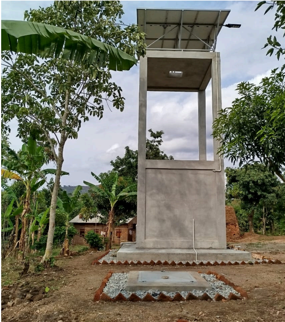
A newly installed solar-powered public water tank in Nangolo, supporting community access to clean water.
