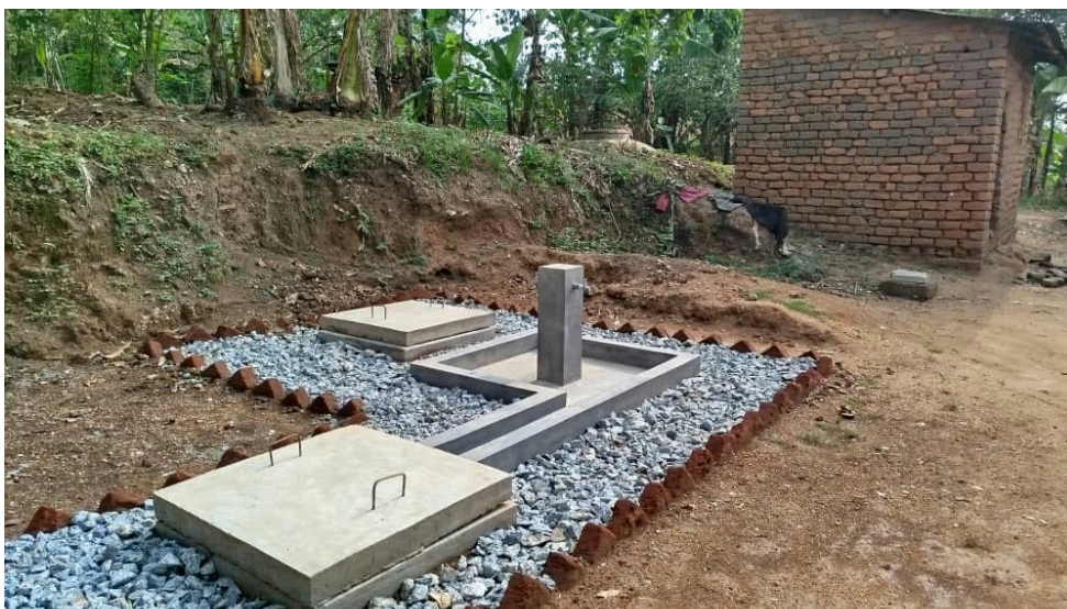
One of several community taps fed by a network of underground water pipes.
