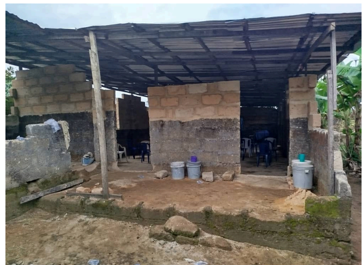
An exterior view of the synagogue building currently under construction, supported by donations from the Initiative for Progressive Judaism Development (IPJD). The ongoing work includes raising the walls, installing doors and windows, adding a ceiling, and providing seating for the worship space.
