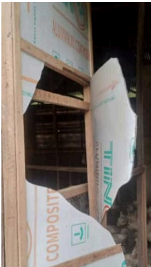
Damage to the poultry facility's entrance following a nighttime break-in by thieves.
